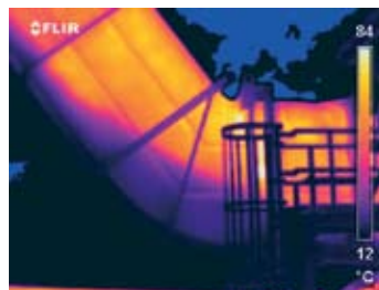
A sediment line is identified in a process plant ducting.
